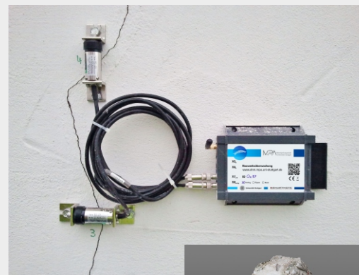
Instrumented crack monitoring with wire-less sensor nodes
