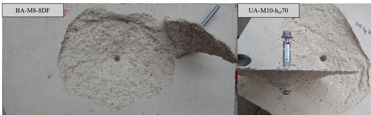
Fig. 2: Brick breakout failure with bonded anchor (left) and undercut anchor (right) [9]
